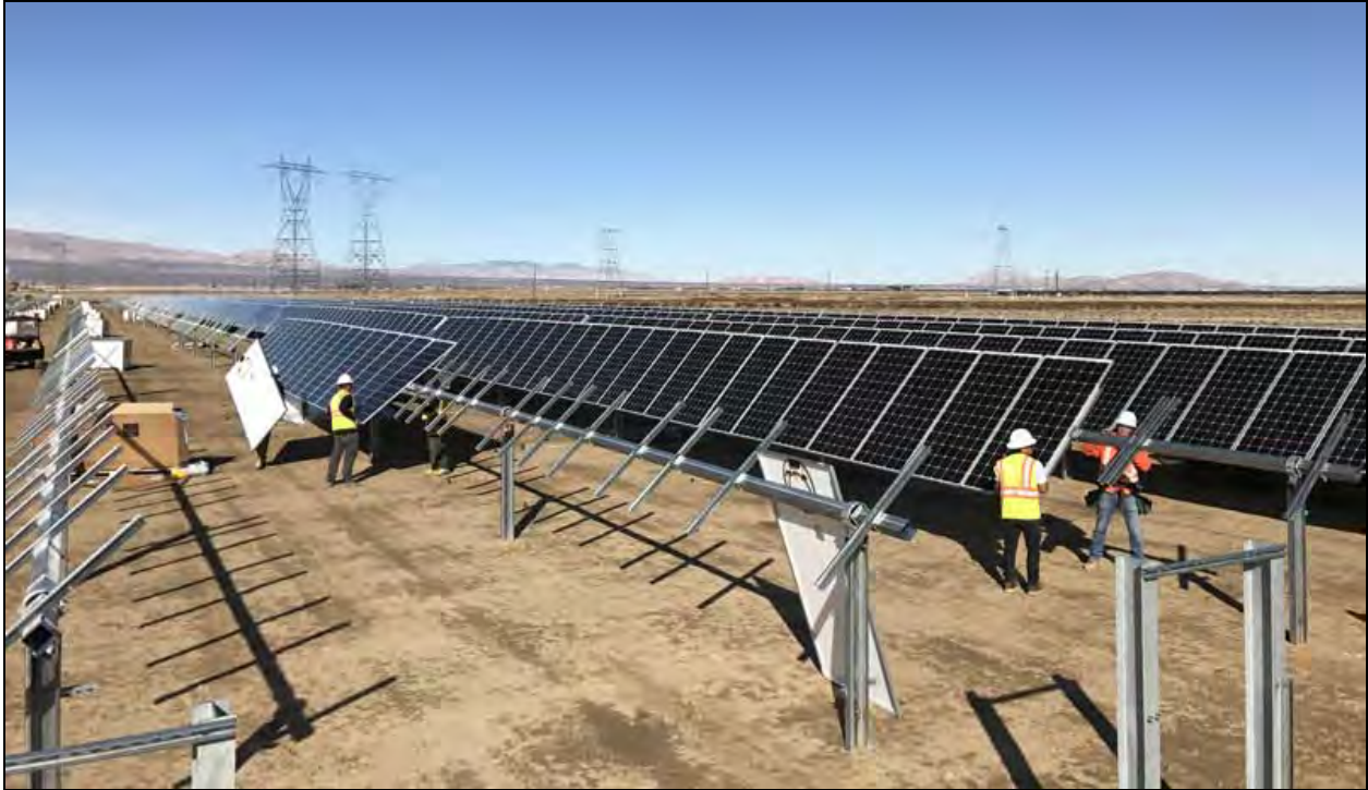
Inset 2. Installation of photovoltaic panel array on steel support beams (Photo: PV Magazine).
