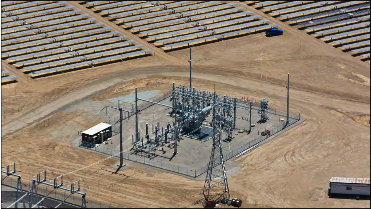
Inset 3. Substation surrounded by photovoltaic panels (Photo: Greentech Media).
