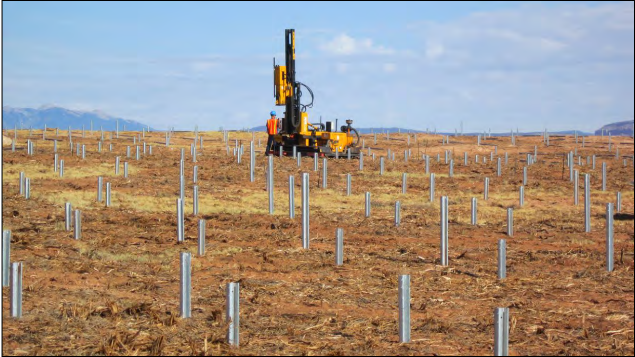
Inset 1. Typical steel support beams for photovoltaic panels and pile-driver during construction (Photo: Clean Energy Collective).
